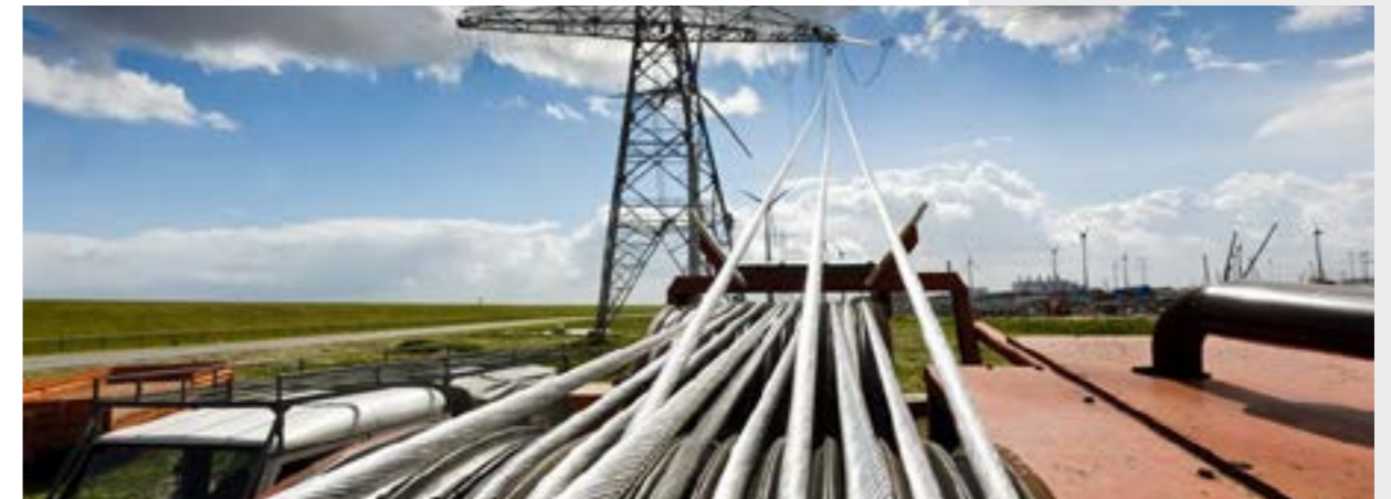
Figure 2: Installation of new high voltage transmission lines to secure power transmission within the system.
