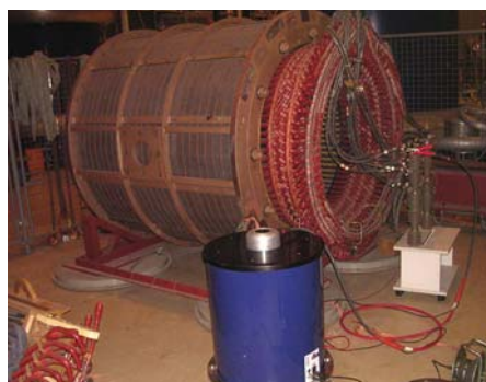
Figure 6b: 30 kV DAC test set (blue) connected to a 23 MW stator. The system is remote controlled using a laptop.
