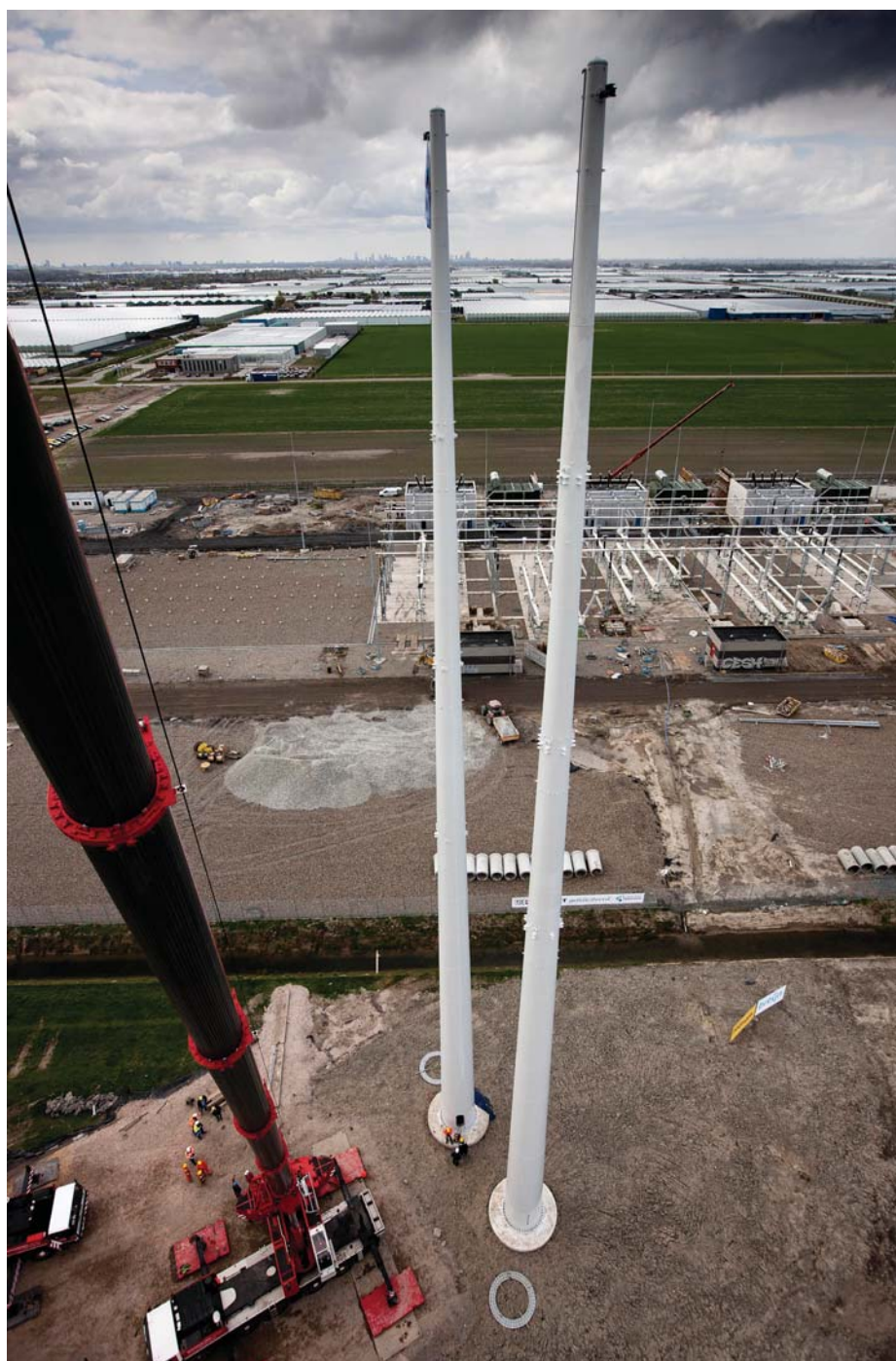
De Wintrackmasten in Bleiswijk
